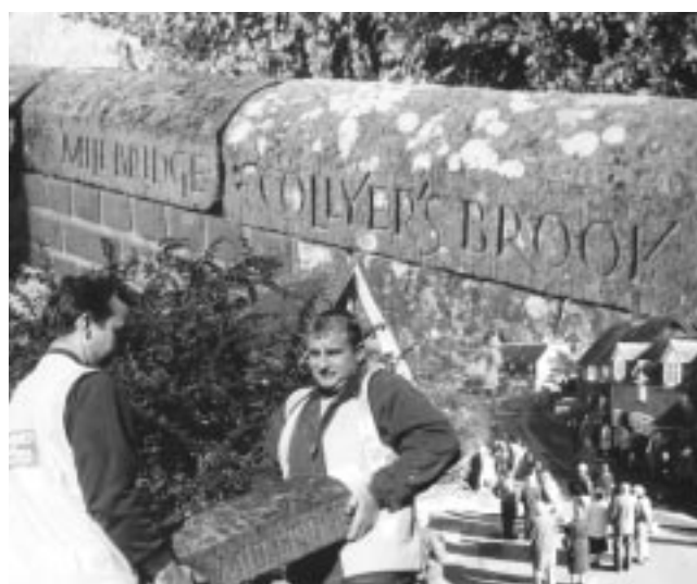
Launching the idea: Angelo Ferrari and Karl Breddy (Dorset County Highways Dept) put into place named bridge stones in Fontmell Magna, Dorset, in October 1999. The letter cutter was Richard Grasby..
